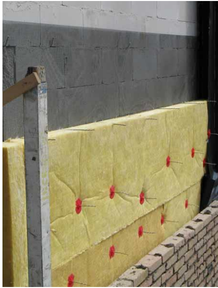
Fig.6. Brick wall construction and filling: (from left to right): white calcium blocks, G-ES netting, mineral wool insulation, 4 cm space, outer brick wall layer.
