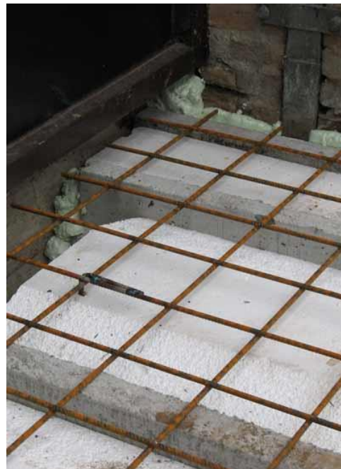
Fig. 9 Reinforcement of concrete floor with steel mats, welded together at some points. Note that small piece of rod pointing downwards for an earth connection, if so
