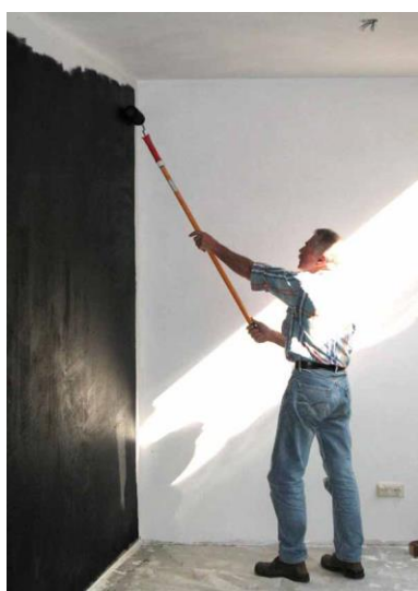
FIG. 10. Painting the wall black with two successive layers of Caparol, using a roller brush.
