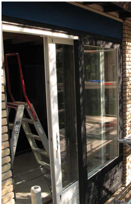
Fig. 8 Treatment of wood with HSF54 paint. Two solid layers (one of the sliding doors) are next covered with two finish layers (not shown yet).
